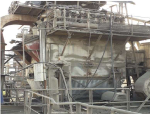
Coal Mill Venting Bag Filter
