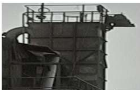
Coal hopper De Dusting Bag filter
