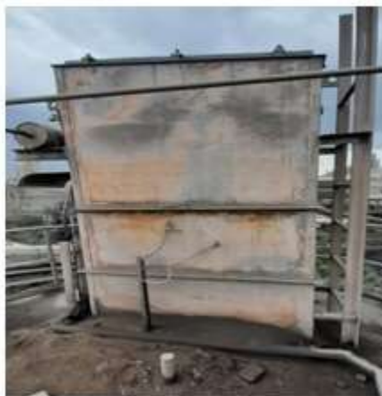
Bed Ash Silo Bag Filter
