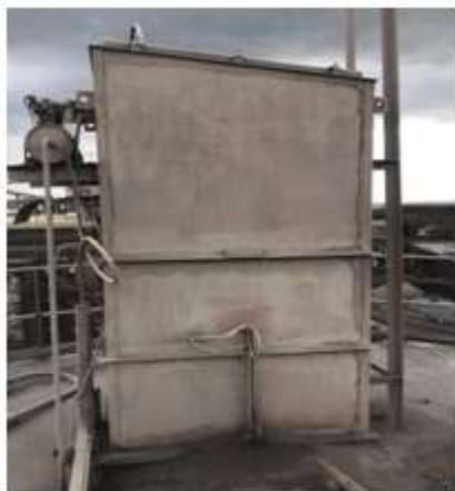
Fly Ash Silo De dusting Bag Filter
