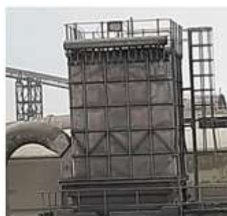
Coal Transfer point Bag filter
